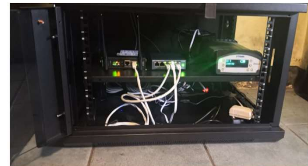
Equipment of the monitoring station at point 8106
